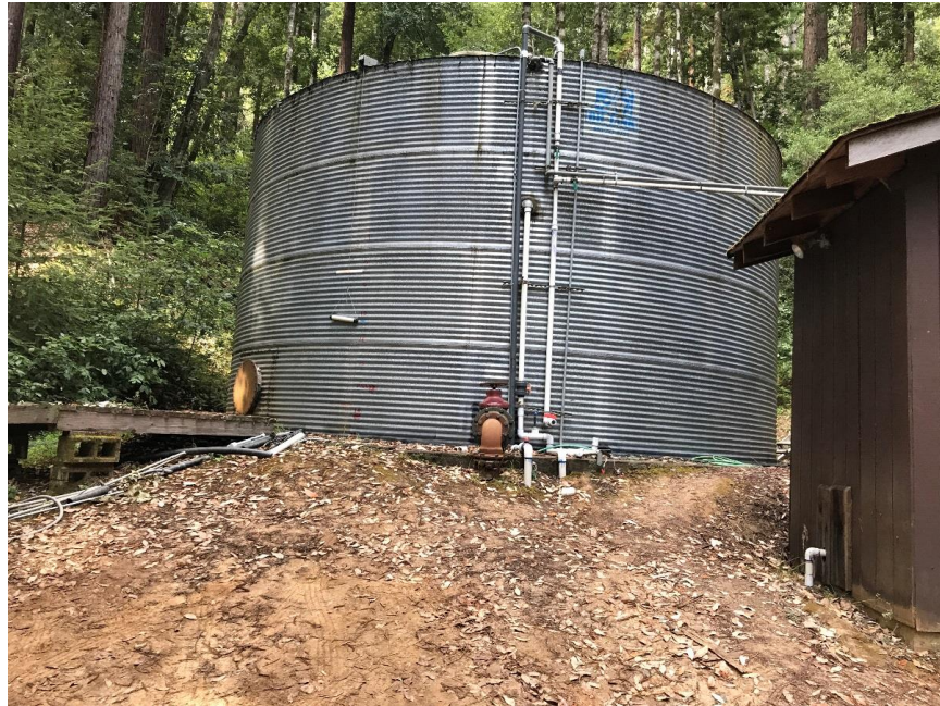
Photo 3. The 70,000-gallon raw water storage tank.
