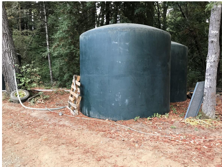
Photo 2. Existing raw water storage tanks at the water infrastructure site.
