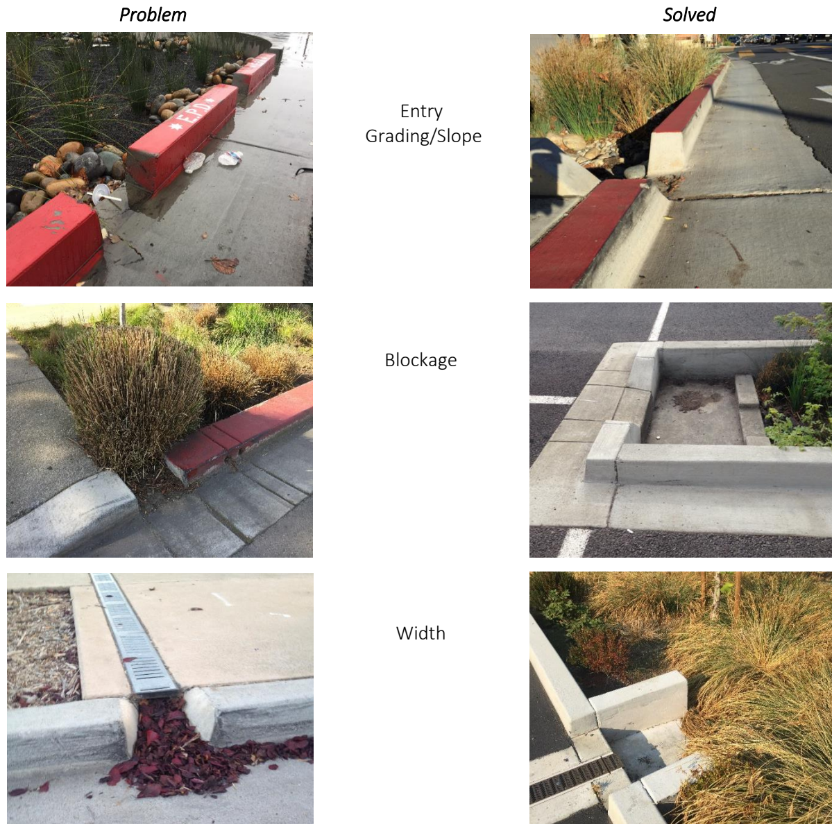
Figure 5-8 – Examples of common design problems with inlets of treatment measures. (Credit: EOA, Inc. and City of Mountain View)
