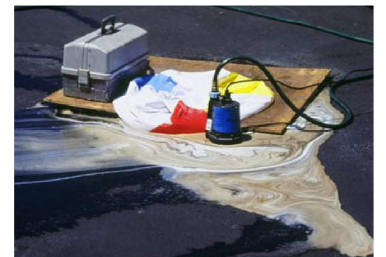
Storm drain inlet is blocked to prevent prohibited discharge. The water must be pumped and disposed of properly.
